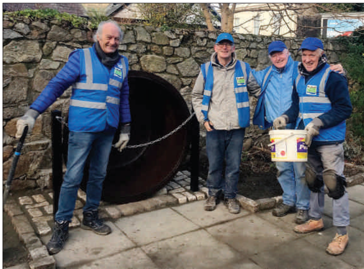
Dalkey Tidy Towns team installing the Famine Pot - Michael, Simon, Des and Frank
