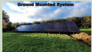
Ground Mounted System
