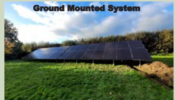
Ground Mounted System
